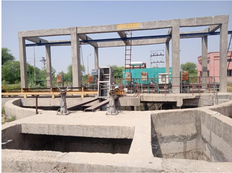
Figure 10.2A: STP located on Suratgarh-Padampur Bypass road, Sri Ganganagar @10.0 MLD Capacity (Latitude & Longitude 29.881490, 73.864333)
